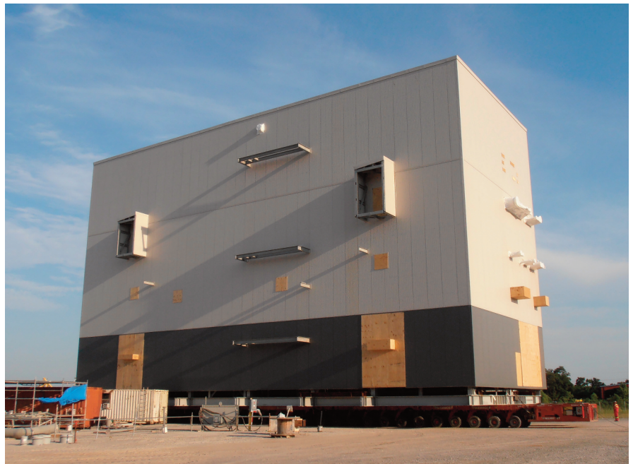
Vale and its partners spent nine years moving some 600 modules like this one from fabrication plants over water, then three kilometres on SPMTs to reach its nickel processing plant in Newfoundland.
